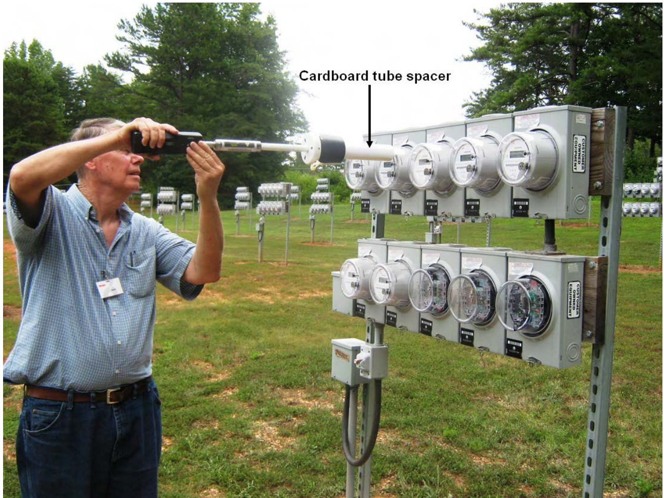
Figure 9-4 Use of the broadband field probe with a cardboard spacer attached to the probe near meters in a rack of ten meters.
