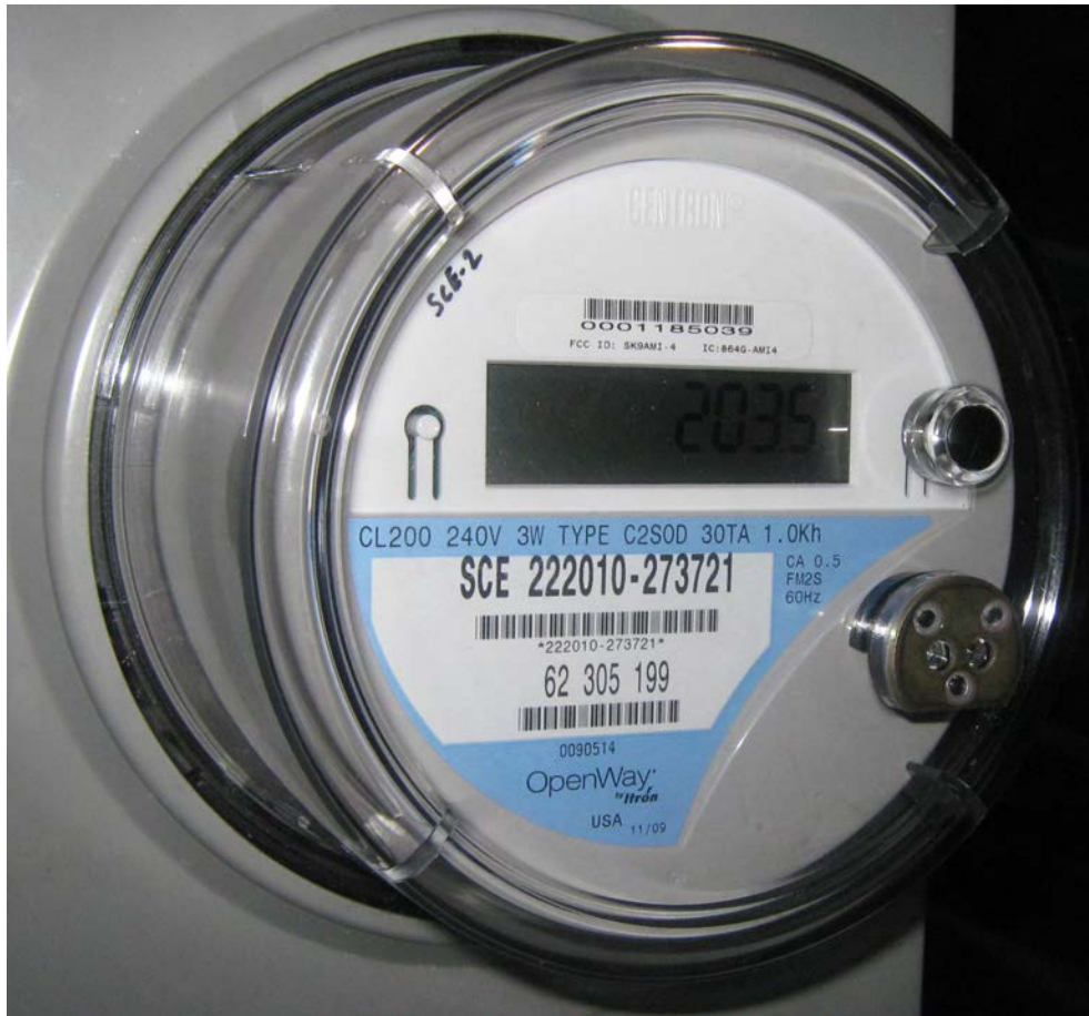
Figure 2-1 Photo of Itron Smart Meter.
